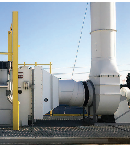
- Air processing system
